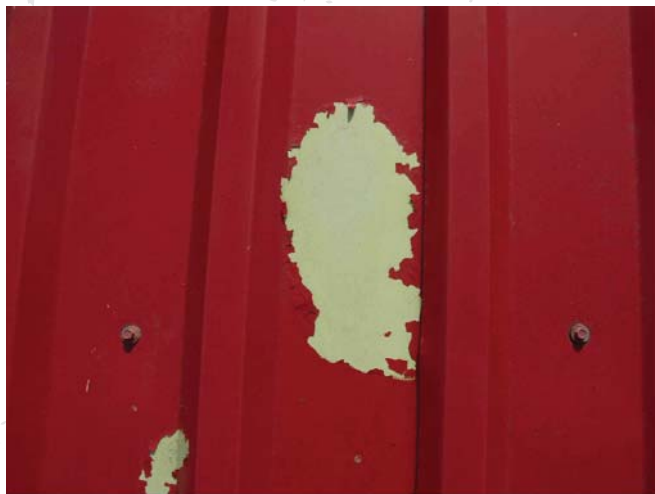
Peeling and flaking of paint is a sign of poor film integrity.
