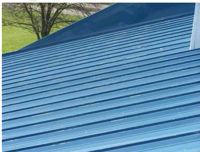
A quality coating system will maintain its film integrity over the life of the structure. This roof is an example of one that is failing.
