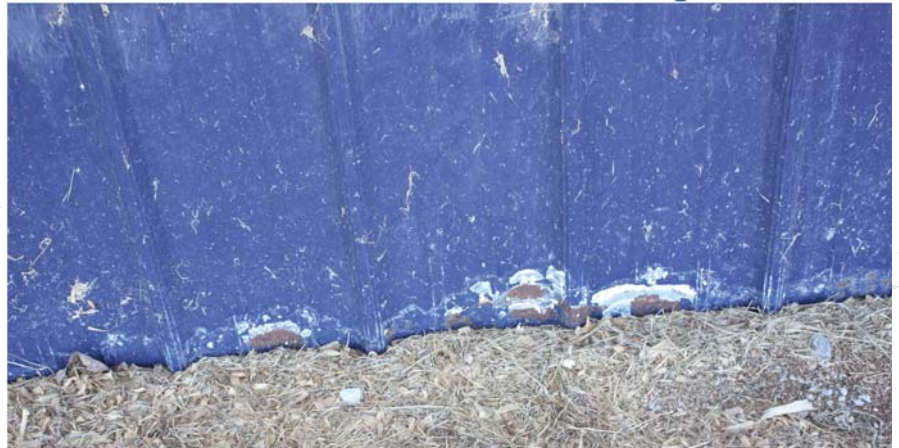
Animal confinement facilities are highly corrosive environments. Care is needed in the proper selection of paint systems, and installation procedures to limit damage.
