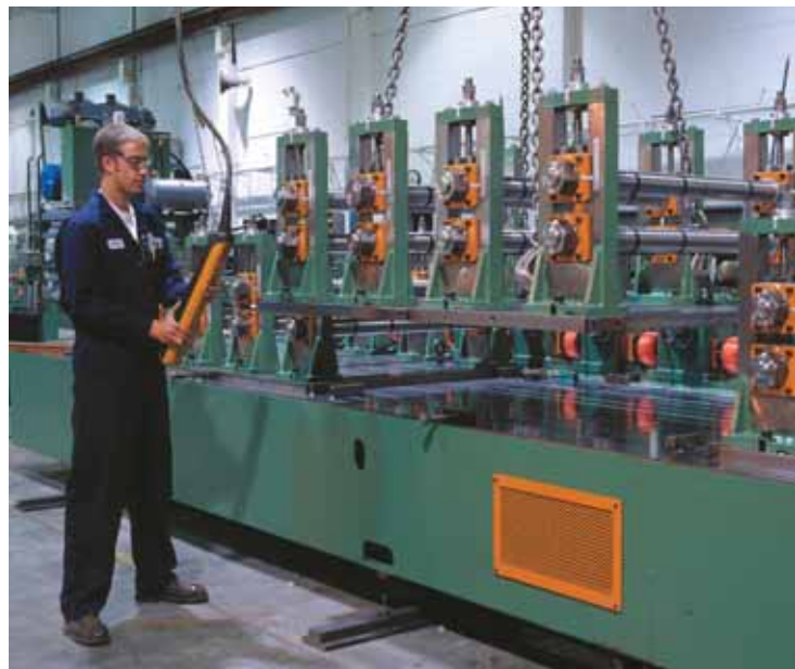
Sets of tooling, positioned on plates, are raised and lowered into place with the push of a button.
