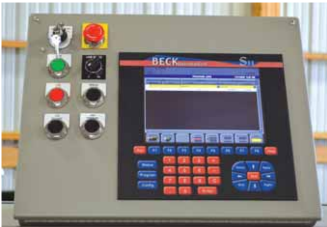
Production is handled with ease via a control panel from Beck Automation.
