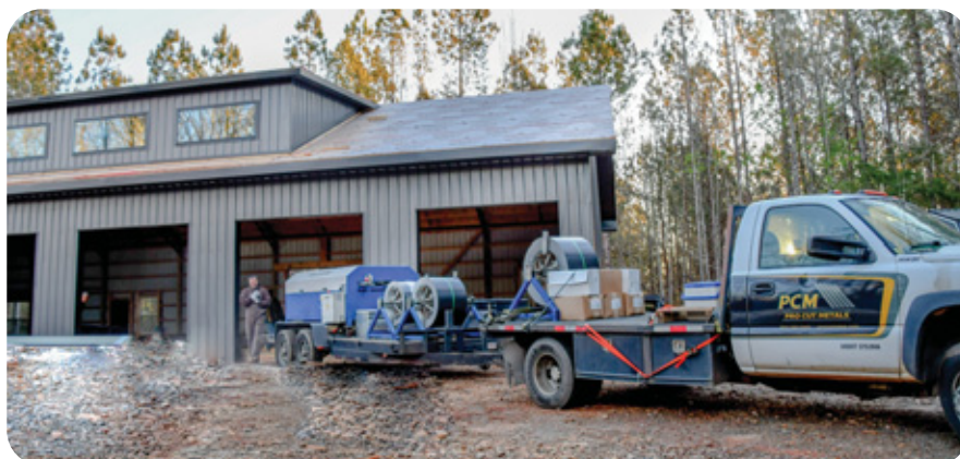
A Schleich Quadro portable roll former is used to make standing seam panels on the jobsite.
