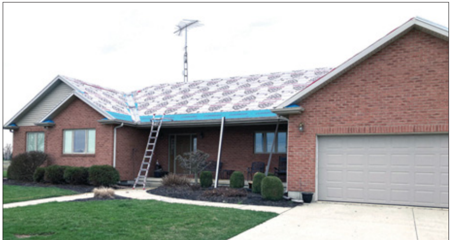
A new standing seam metal roof is replacing asphalt shingles on this home near Sidney, Ohio.
